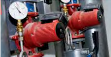
Actuators, valves, control cabinets
