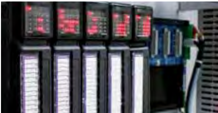
Connections to PLC
